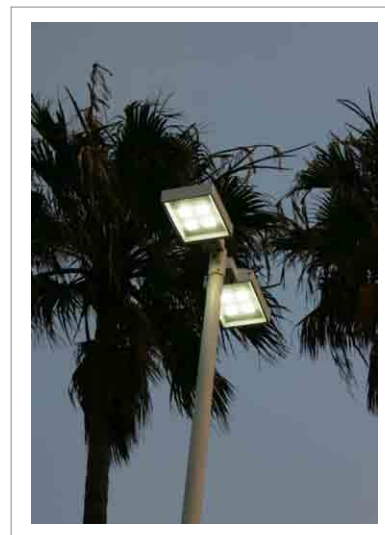
Figure 1: LED street lights
