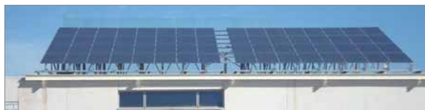
PV installation and control system at the University
