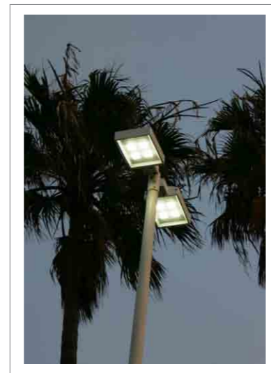
Figure 1: LED street lights
