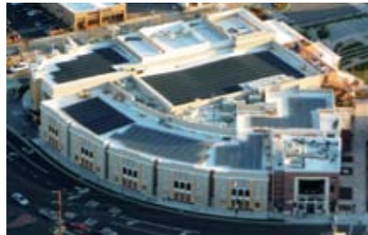
132 kWp system by SPG Solar, Inc., on the rooftop of Cinema West's Livermore Cinemas in Livermore, CA.
