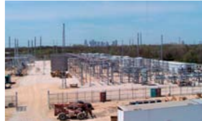
Parkdale substation in the Dallas-Fort Worth area.
