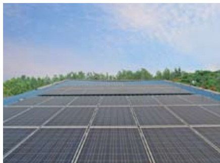
The installed solar panels at the Goethe-Institut, Bangalore
